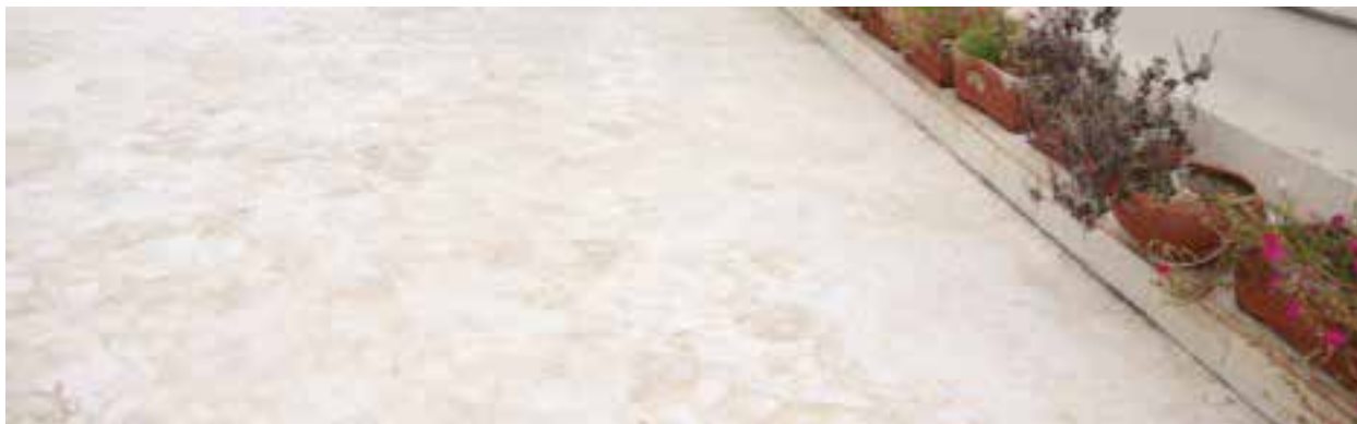
Close-up of the white rooftop materials used to naturally keep the Legacy Spectral building cooler by reflecting light and heat.
